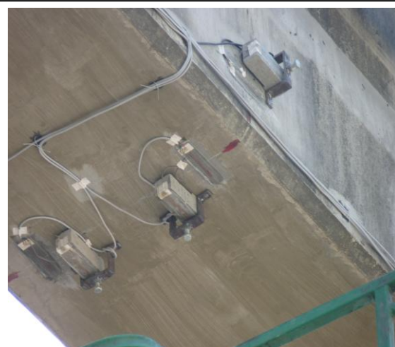
Strain gauges and Wiring
